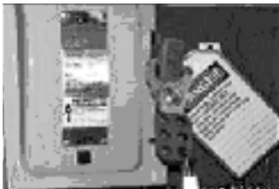
Always lock out and tag out circuits.
