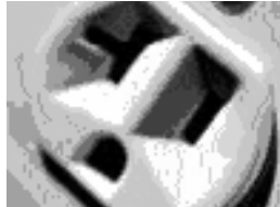
Outlets must be grounded properly.
