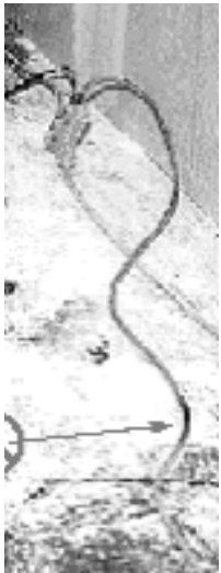
This extension cord is damaged and should not be used.
